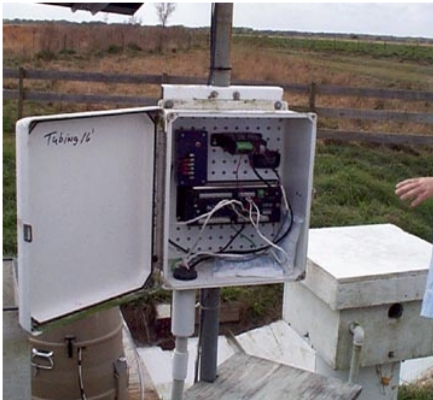
Figure 3.10. Datalogger/controller shelter and hardware.
