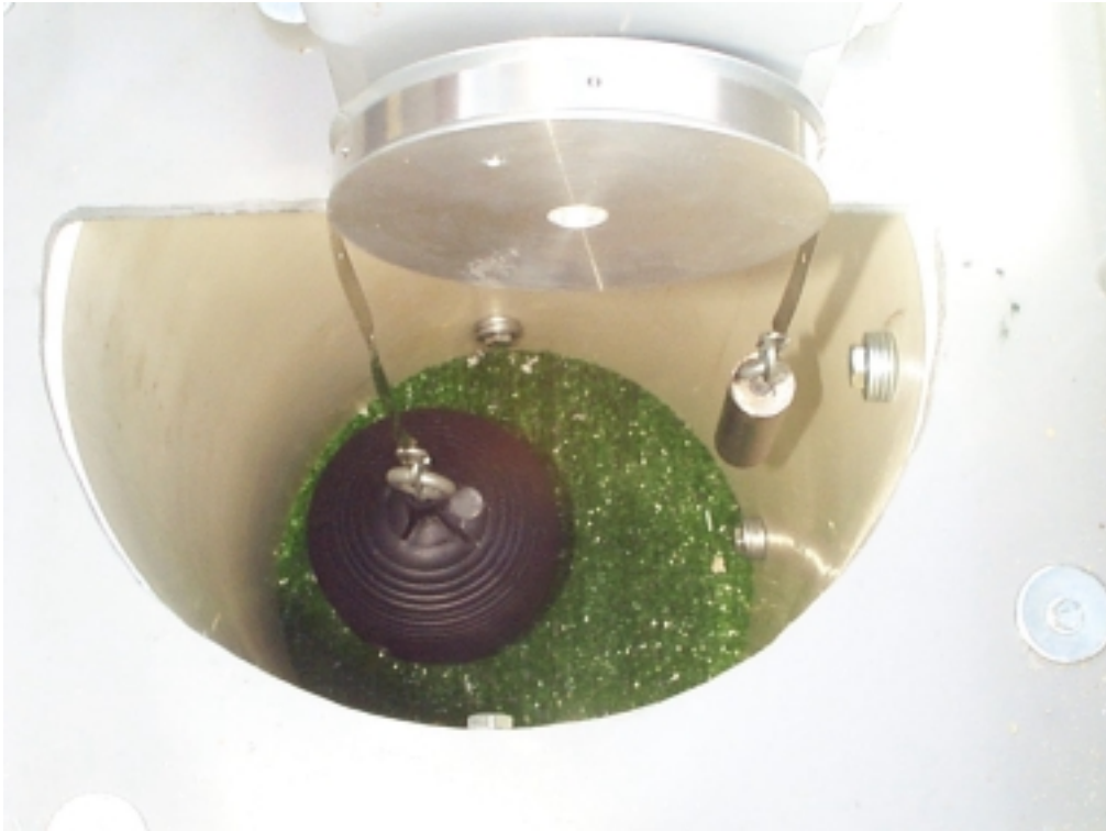
Figure 3.8. Stilling well with pulley, float and counterweight.
